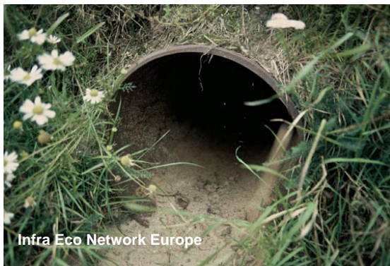
Figure 60. Pipe culvert designed to accommodate small mammals.
