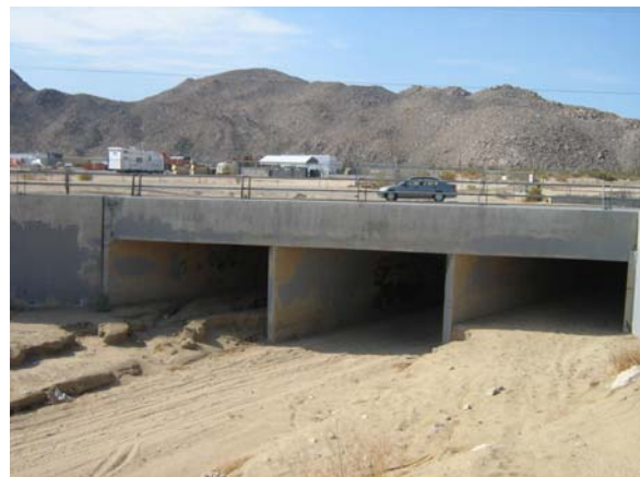
Figure 62. Looking south towards Joshua Tree National Park at the structure for Quail Wash on Highway 62.
