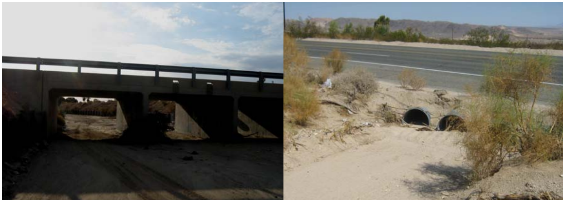
Figure 65. Bridge for Savahia Peak Wash on Highway 62 (left), and pipe culverts under Highway 62 near Shoshone Valley Road (right).
